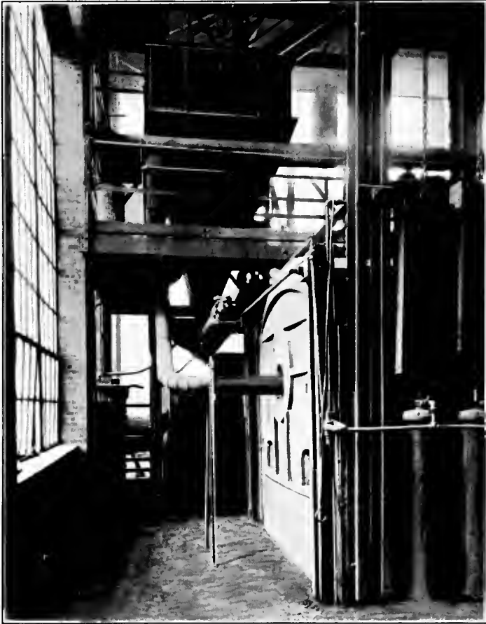
FIG. 102.—Fuller No. 201, Burner and Coal Bin.
